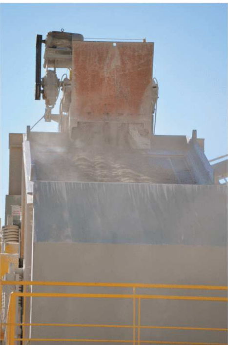
Somerset Stone's finish screen uses Major Wire's Flex-Mat 3 Tensioned on all three decks to make #11s (5/16-in.), or Class I sand and lime.
